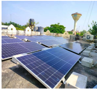
4) Shopping Complex – 30 KWp
