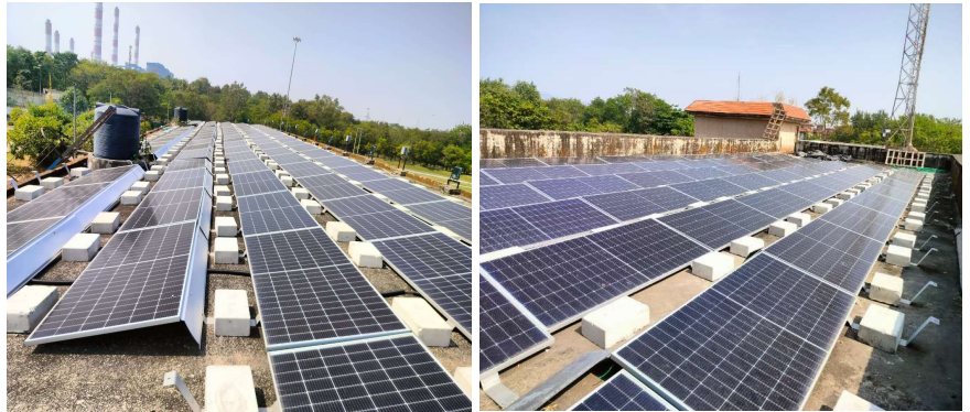
1) Stadium gallery – 40 KWp
