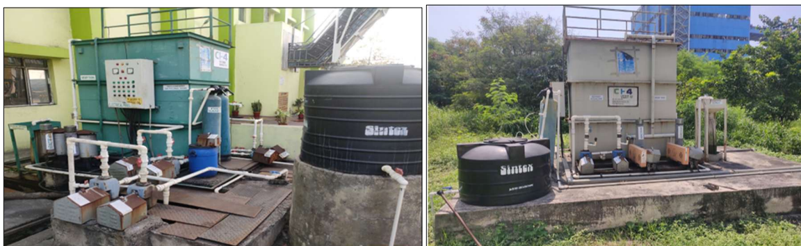
Fig 3 Pre Fabricated STPs operational at 18 locations of NTPC Sipat
