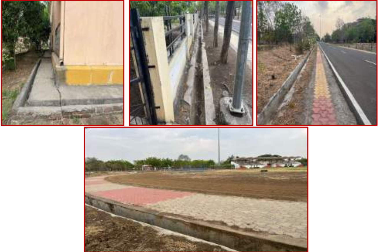
Plate 47-50: Rainwater harvesting structures in NTPC Solapur
