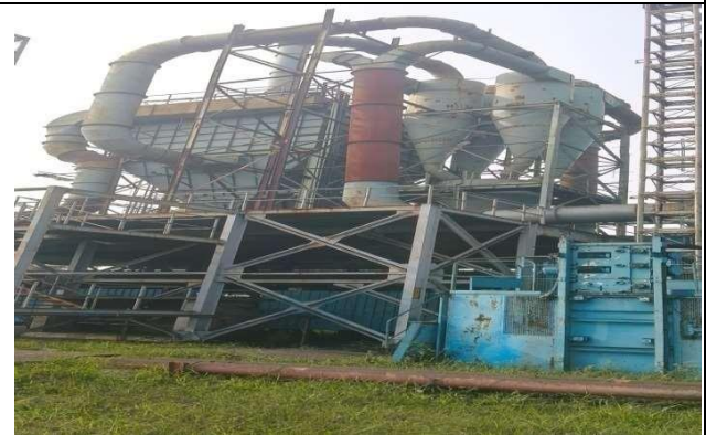
Dust extraction system at coal crusher house.
