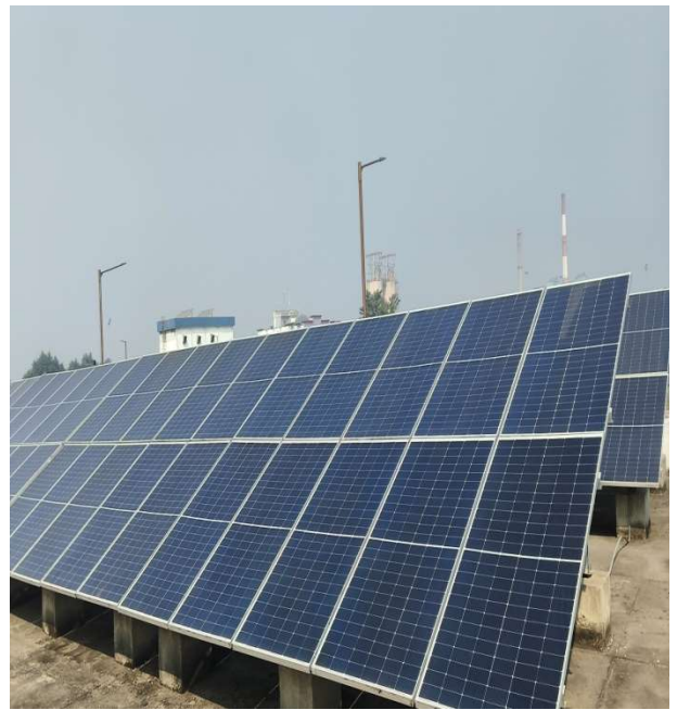
Roof top solar systems at Switch yard room roof
