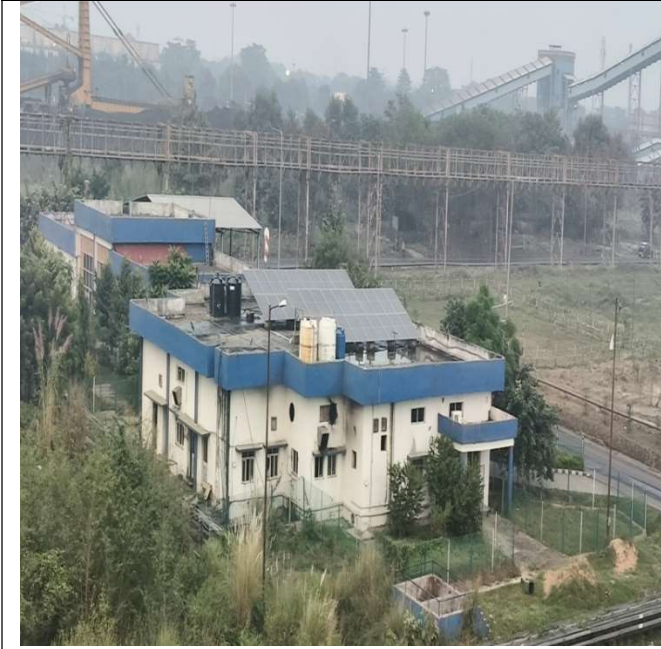
Roof top solar systems at canteen
