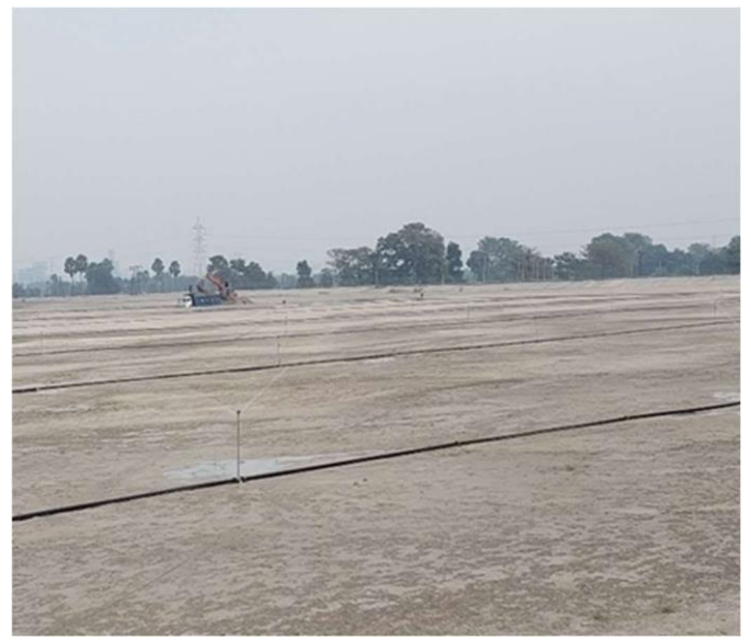
Mechanized Water Sprinkling Network
