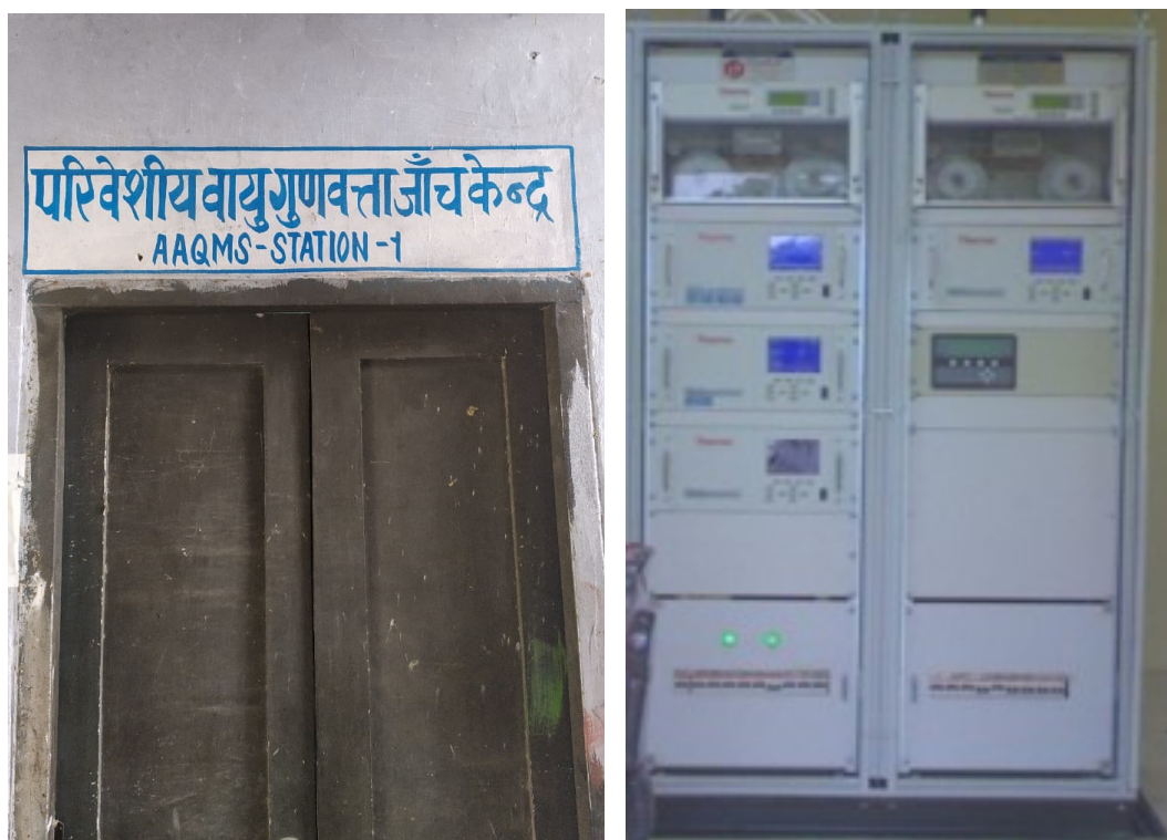
Continuous Ambient Air Quality Monitoring Station
