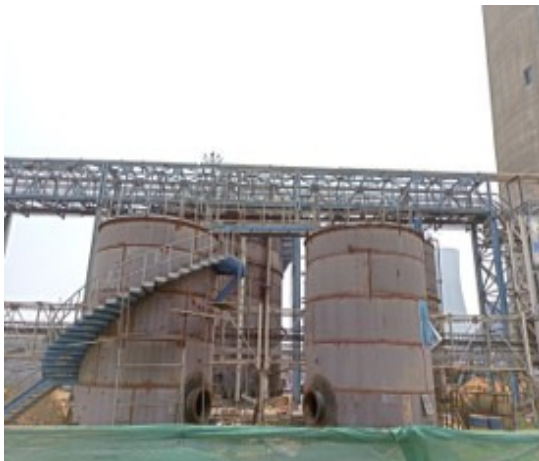
(Storage and Process Water Tanks)
