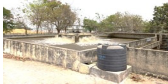
(Sewage Treatment Plant at Township)
