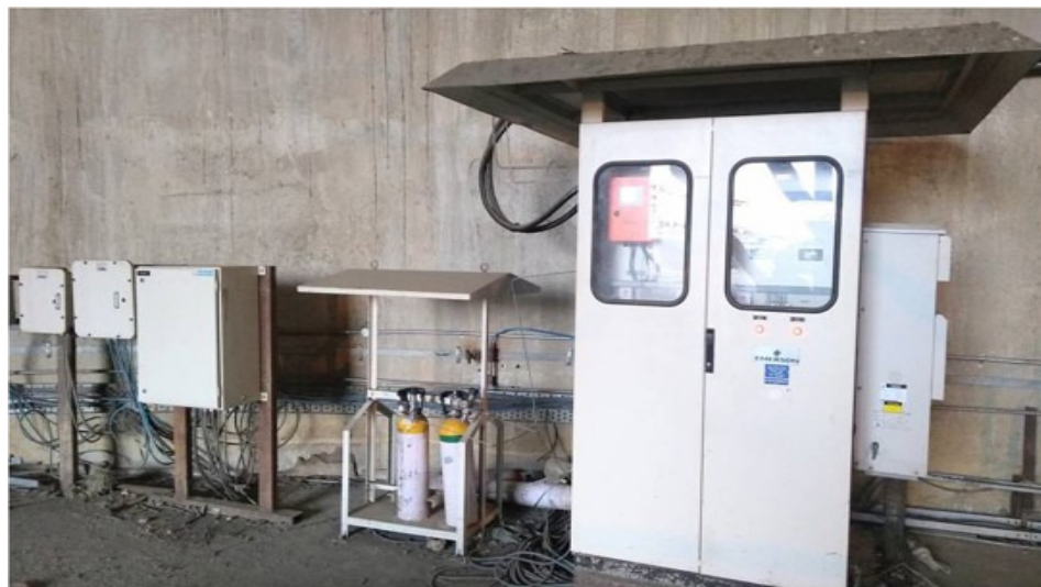
Continuous Emission Monitoring System
