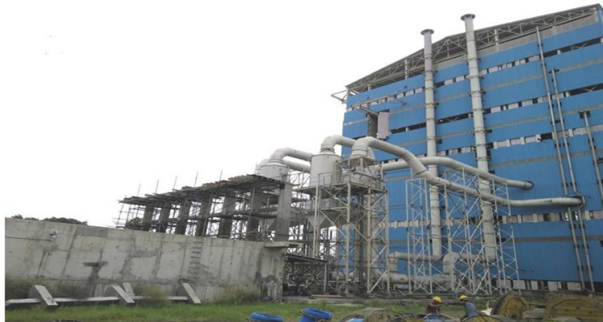
(Dust Extraction Dust Suppression at Crusher House)
