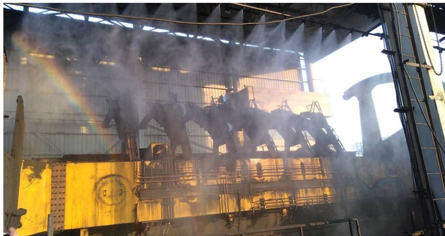
(Dry Fog Dust Suppression System at Wagon Tippler)
