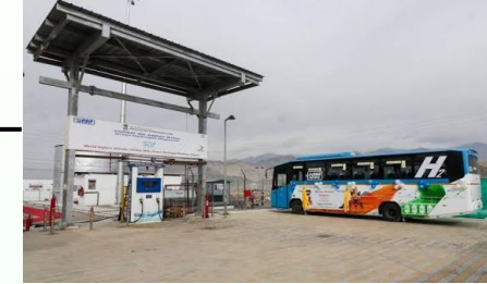
80 Kg/Day H 2 Generation, 5 nos. Fuel Cell Bus, Leh, Ladakh
