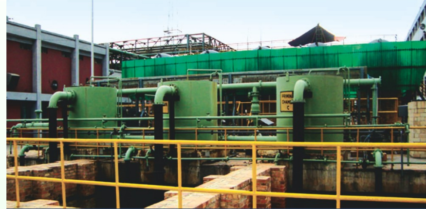
Neutralization Pit at DM Plant
