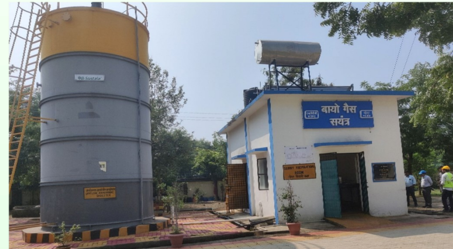
Bio-Gas Plant at NTPC
