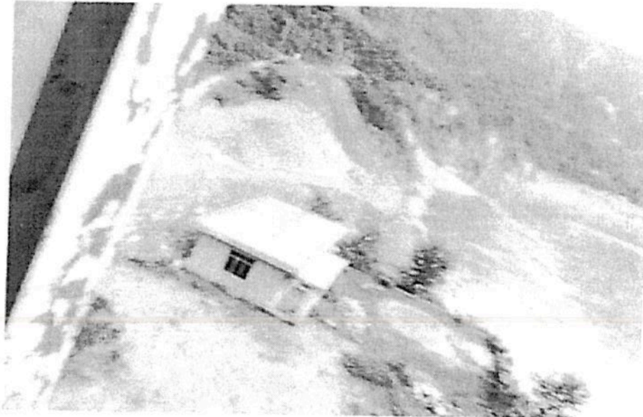
6. LHS River Satluj: Opposite spillway plunge pool , provided protection found washed out.
