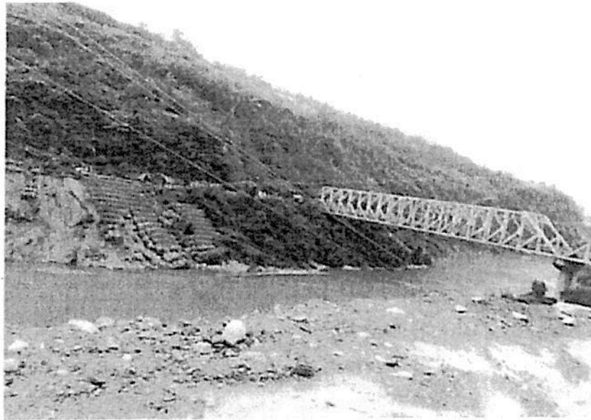
1. Damaged protection works near Maitri Setu LHS of River Satluj.
